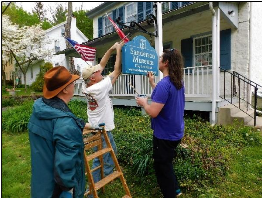
Our Curator, Chuck Ulmann, observing the installation of our new front sign by Volunteer Stephen Pierce.
